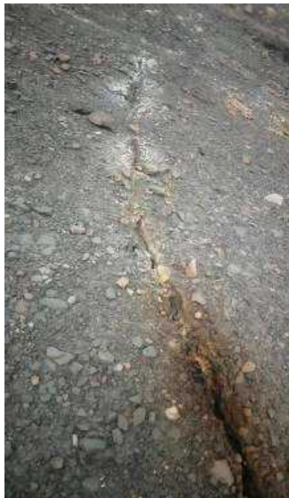
Figure 20: Fume cracks in the Bhulanbarari area.
